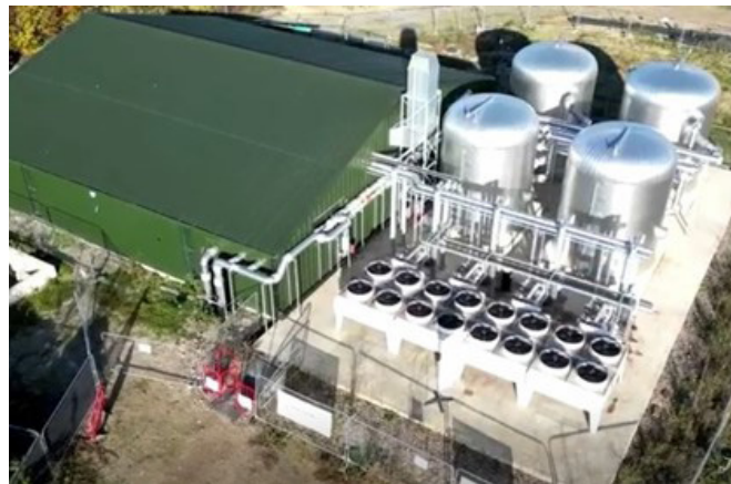
Figure 2: Energy Centre (left) and Thermal Stores (right)
