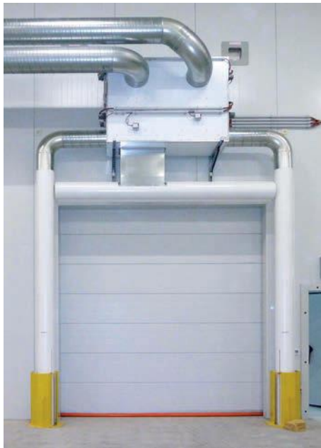
Figure. 3 View of air separation on the inside of a cold store doorway
