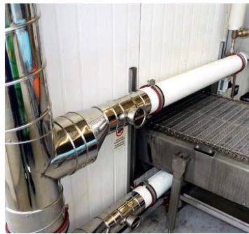
Figure. 4 Air separation at a blast freezer
